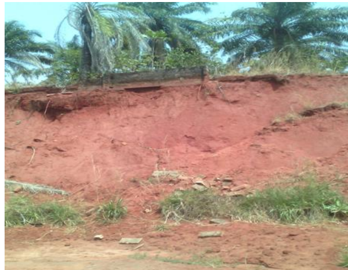
Plate 1: Showing the collapsed walls of Doro Gardens due to sand mined activities
