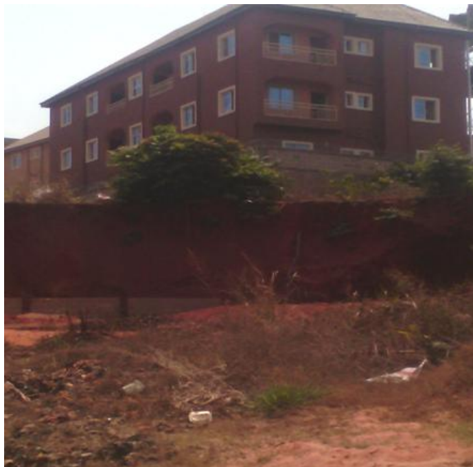
Plate 3: Showing a threatened residential building located within the mined area.
