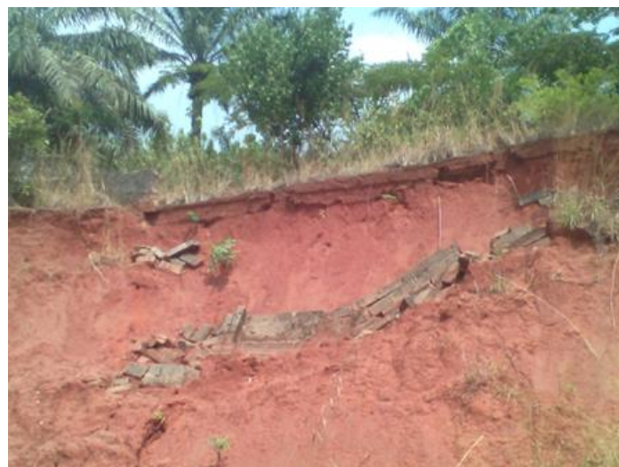
Plate 2: Showing another collapsed fence of the village town hall at Awka North due to sand mined activities.
